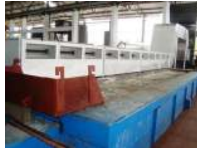
Suction Slot Duct Extraction System
