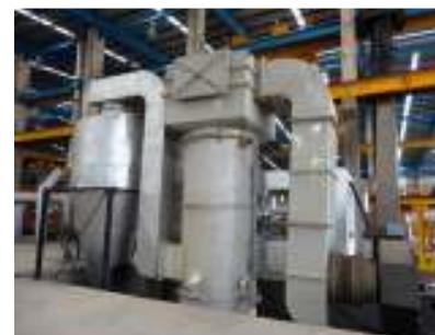
Wet Scrubber with Dust Collecting Cyclone
